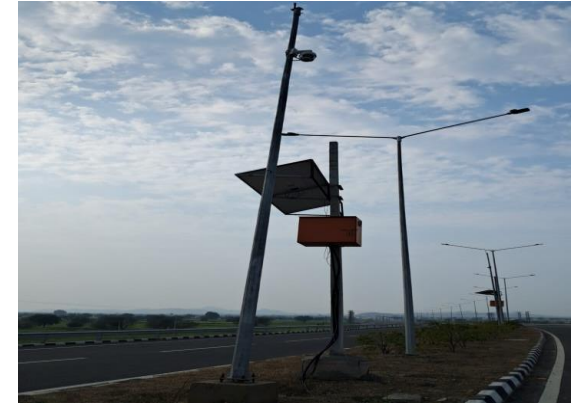
Fig 4.236: Camera with solar panel at Ch 2+250
