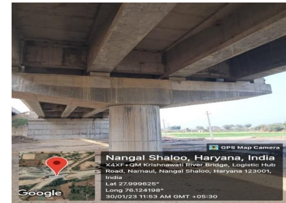
Fig 4.263: MJB at Ch. 2+130
