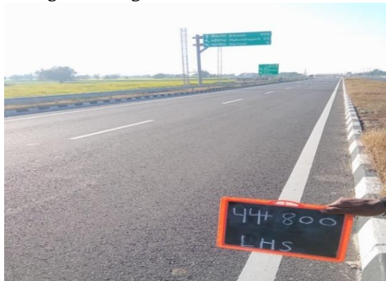
Fig 4.201: Sign Board at Ch 44+800 LHS
