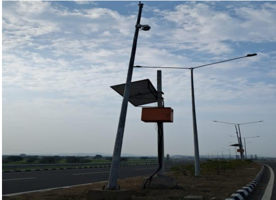
Fig 4.234: Camera with solar panel at Ch 2+250
