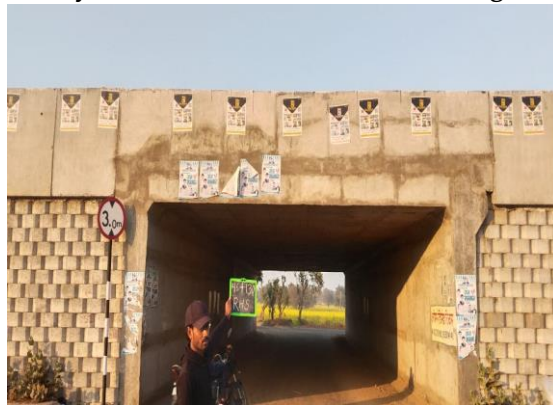
Fig 4.320: PUP at Ch. 32+207 RHS
