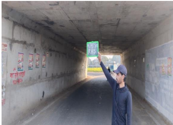
Fig 4.325: PUP at Ch. 47+780 RHS
