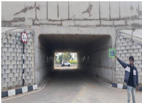
Fig 4.331: PUP at Ch.55+960 RHS
