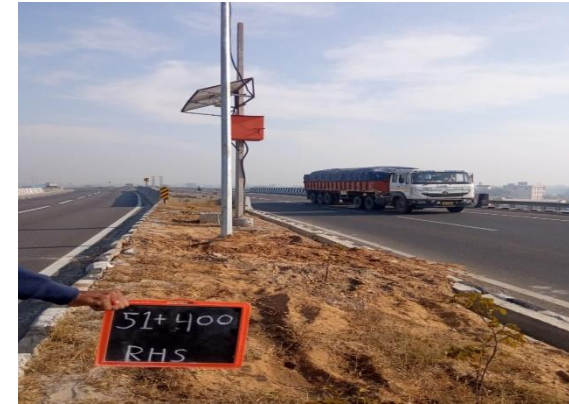
Fig 4.230: Camera with solar panel at Ch 51+400
