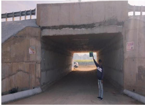
Fig 4.328: PUP at Ch.50+480 RHS
