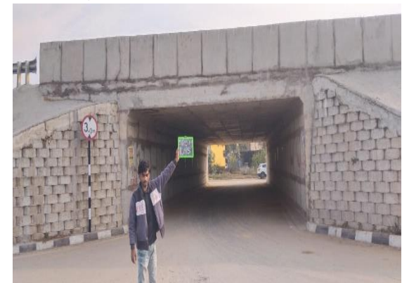
Fig 4.332: PUP at Ch 56+510 RHS
