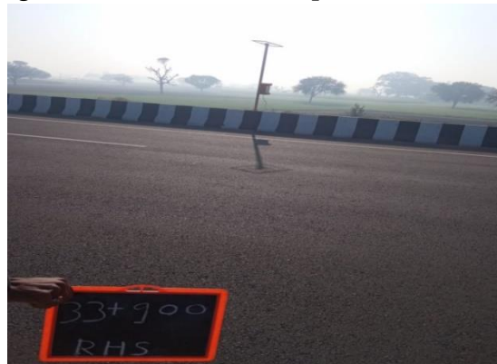
Fig 4.226: SOS Box at 33+900 RHS
