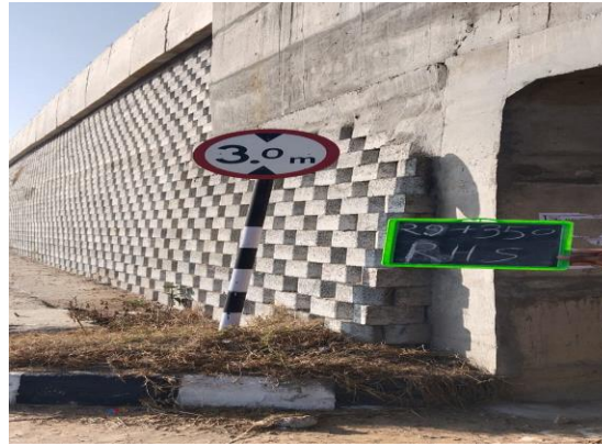
Fig 4.312: PUP at Ch. 29+350 RHS
