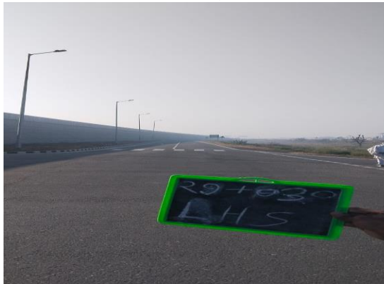
Fig 4.214: Lighting at Ch. 29+630 LHS
