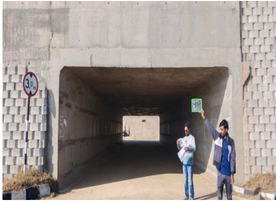
Fig 4.311: PUP at Ch. 29+350 RHS
