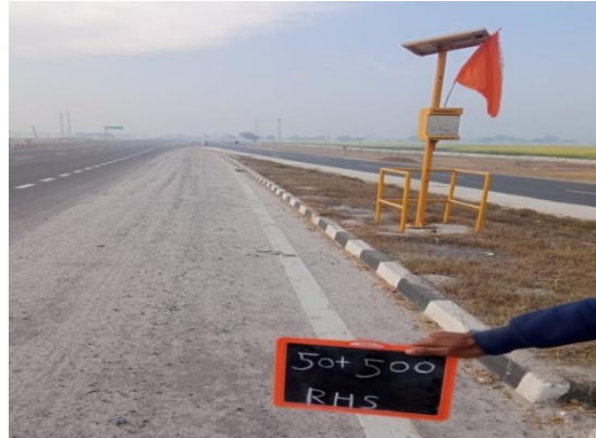
Fig 4.232: SOS Box at 50+500 RHS ILMH
