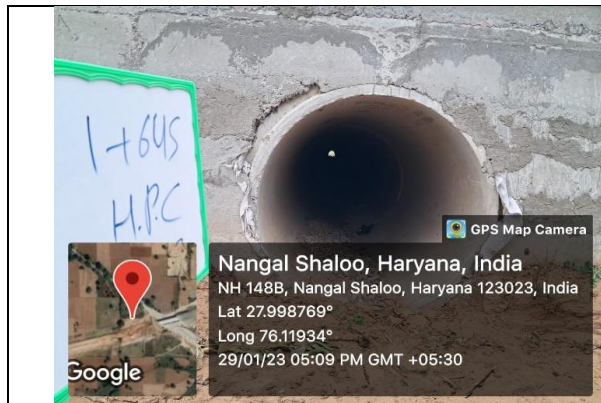
Fig 4.388: HPC at Ch 1+645
