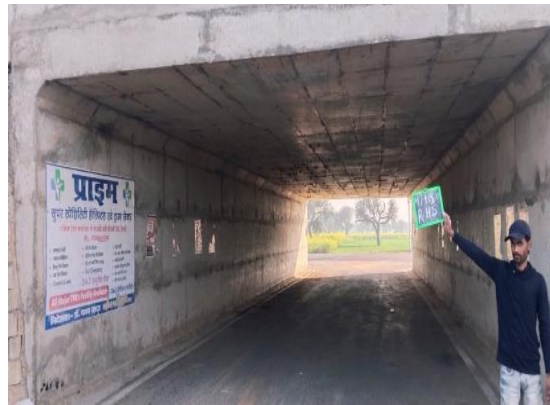
Fig 4.323: PUP at Ch. 47+140 RHS
