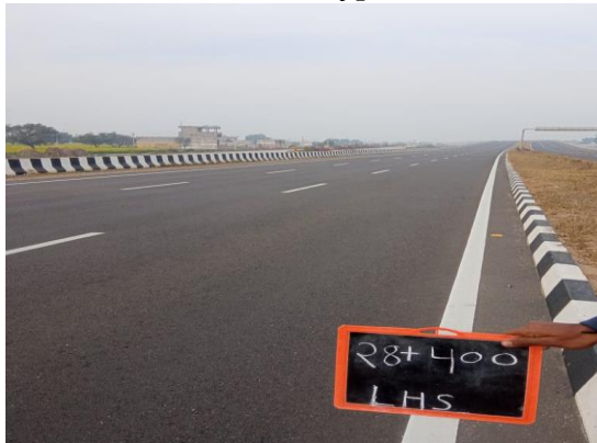
Fig 4.205: RCC crash barriers at Ch 28+400 LHS
