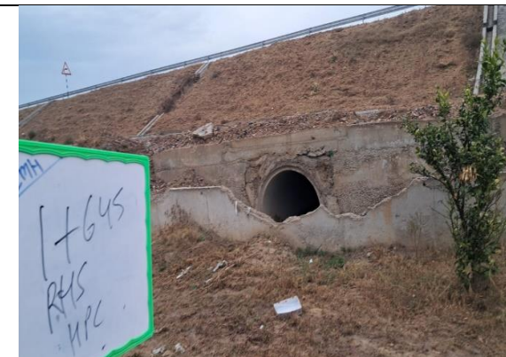
Fig 4.390: HPC at Ch 1+645
