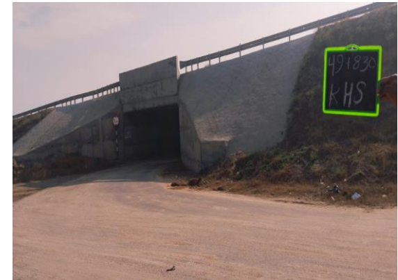
Fig 4.327: PUP at Ch. 49+830 RHS
