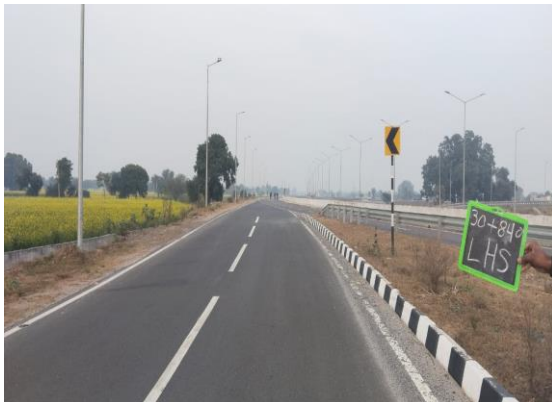
Fig 4.216: Lighting at Ch. 30+840 LHS
