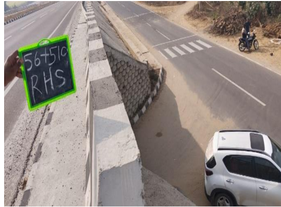
Fig 4.334: PUP at Ch 56+510 RHS
