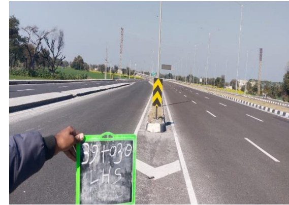
Fig 4.200: Sign Board at Ch 39+030 LHS
