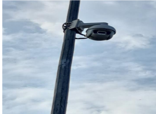
Fig 4.235: Camera with solar panel at Ch 2+250
