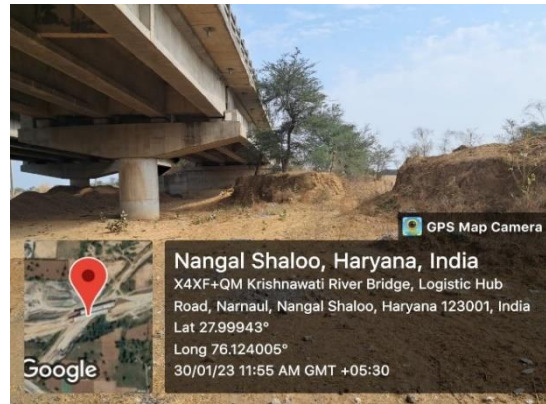
Fig 4.259: MJB at Ch. 2+130
