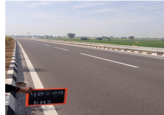
Fig 4.209: MBCB at Ch 48+800 RHS
