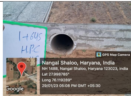
Fig 4.389: HPC at Ch 1+645
